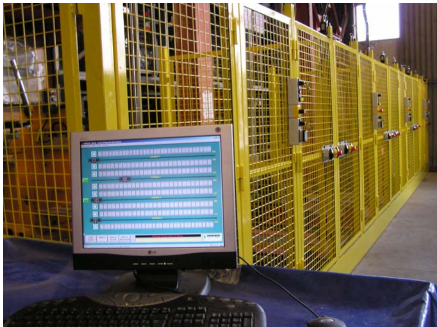
Rik-Fer revamped the warehouse by applying Movicon Supervision to manage it completely in automatic.
