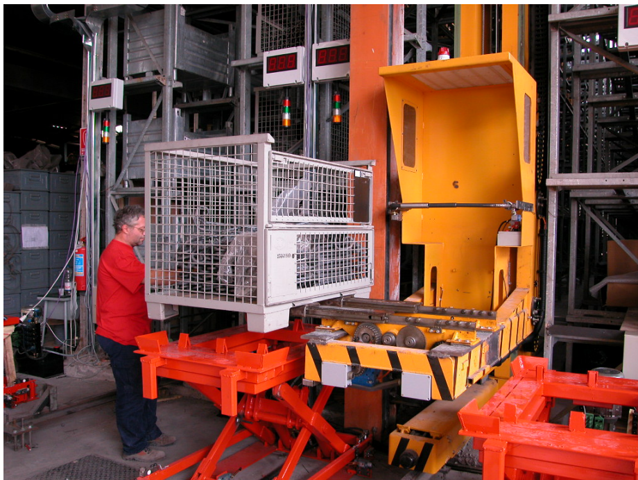
One of the loading/unloading bays. A weighing system makes an exact and precise calculation on goods available.
