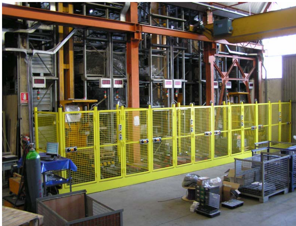
The circulation and storing system of merchandise manufactured by Rik-Fer of Pordenone (Italy) automated by Co.Mar Automation.
