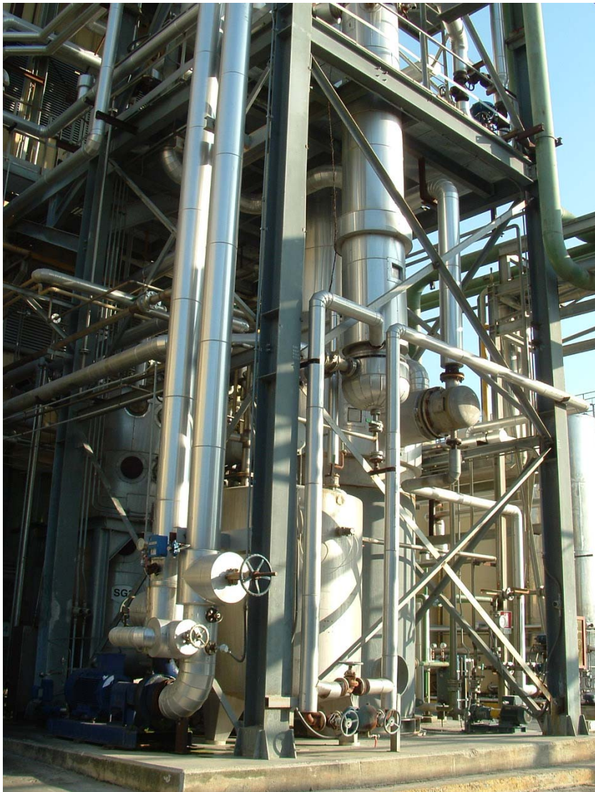
The revamped Fox Petroli biodiesel production plant.
