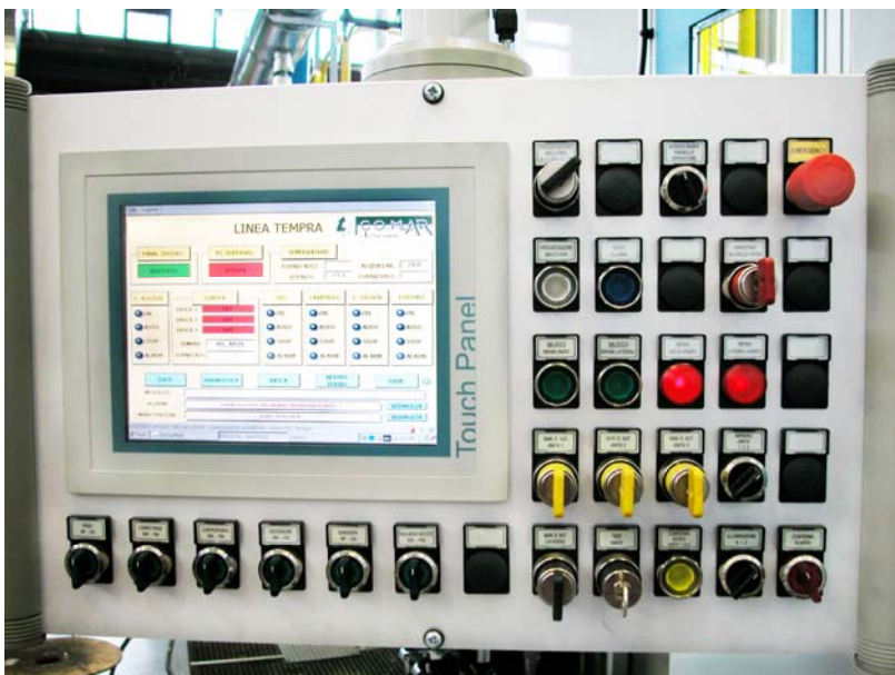
Displayed details on one production line's work substations. Each substation is equipped with an operator control unit and HMI touch panel based on Movicon for Windows CE, connected through LAN Ethernet with the Movicon Supervisor.
