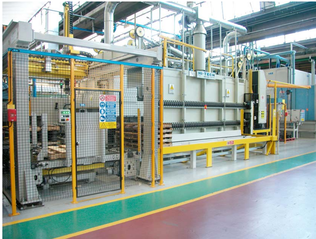
The final Palletization stage in the new roller tempering production line process belonging to the Italian manufacturers of track loader components.
