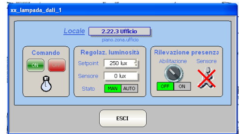
Figure 2 – Control units with detailed information/commands
