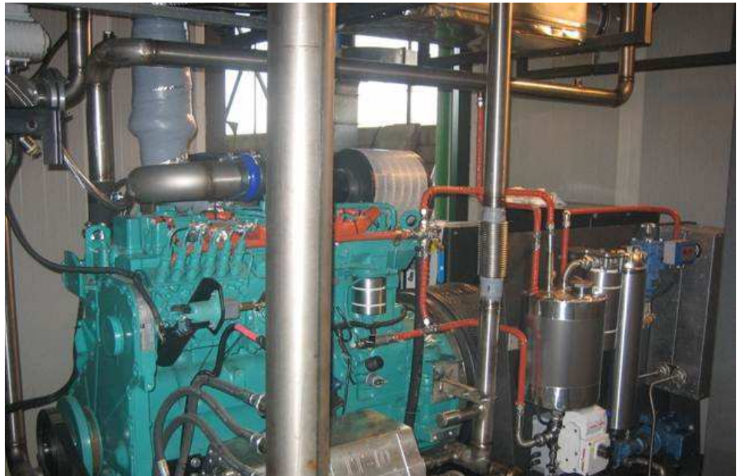
Inside the cabin of a 100 kW electric-thermal energy production generator designed by Powertron. The system works on an average of 650 hours/month continuously.
